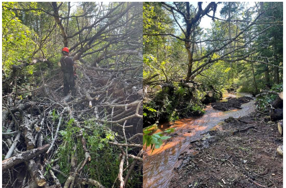
Figure 3. Before and after photo of a large blockage removed by field crew in 2023.
