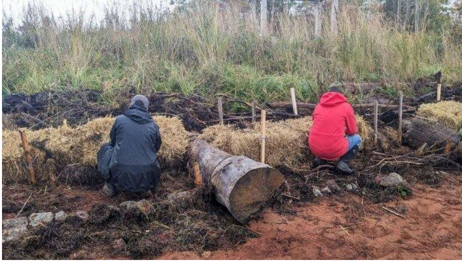
Figure 45. Volunteers work on preparing the living shoreline for the fall and winter storm season. Photo Credit: Shane Hennessey/CBC Figure 46.
