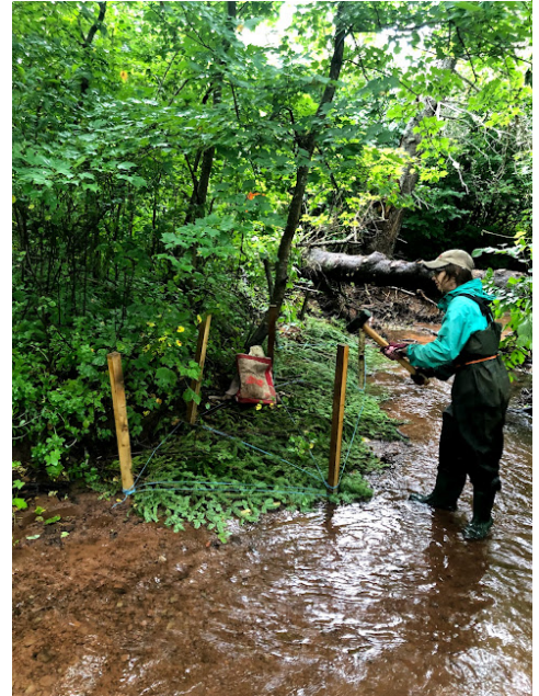
Figure 2. Image of our summer crew member, Teo, hammering in the stakes during brush mat assembly.
